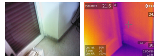
FIGURE 24 - THERMAL LOSSES IN THE WINDOWS AND WINDOW INVISIBLE TO THE NAKED EYE This figure shows the thermal losses due to thermal bridges in the corner of the room.
